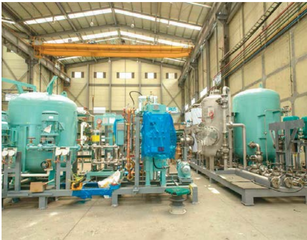
Fresh Water Supply Plant
