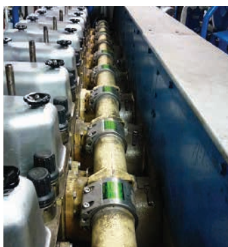
MJG EPDM 100A. engine room. Australia
