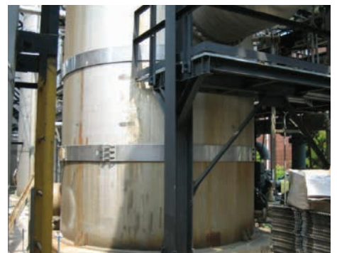
MJFL FKM 3,615mm. incinerator. for supplementation of weld. Korea
