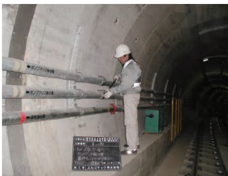
MJGF EPDM 100A. pump up drain pipe. subway station. Japan
