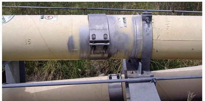
MJS EPDM 400A. mineral conveying line. Australia
