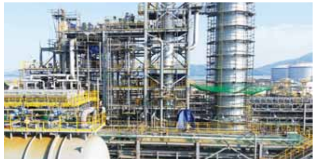
SNG Pipe Insulation
