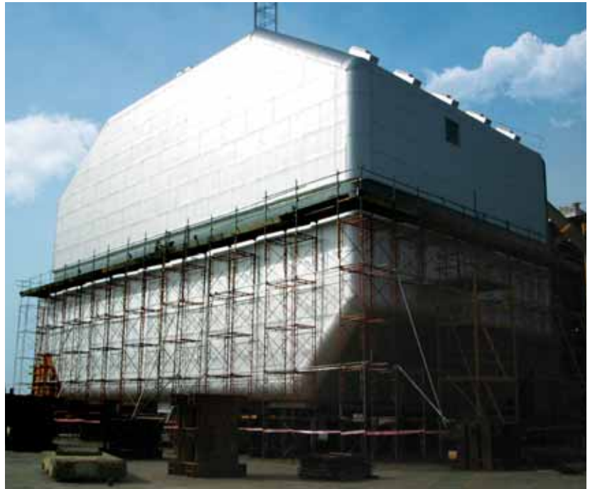
Prismatic Type LPG Cargo Tank Insulation
