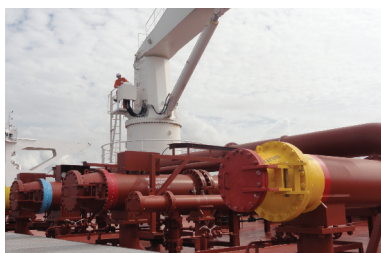
• Hose Handling Crane Cylinder
