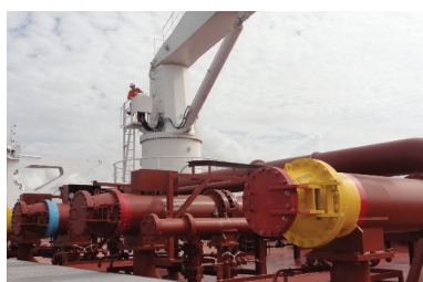
• Hose Handling Crane Cylinder
